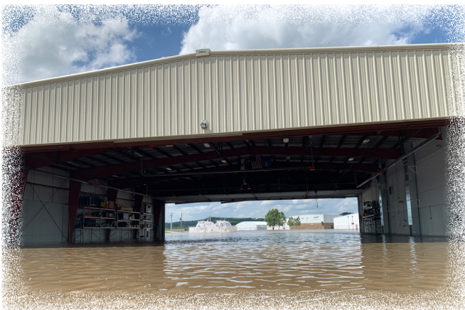
At the height of the flooding, nearly five feet of water stood in the abandoned Patrol hangar.
